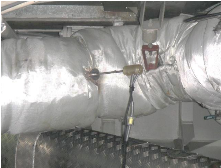
Figure 6. Exhaust gas sampling point
