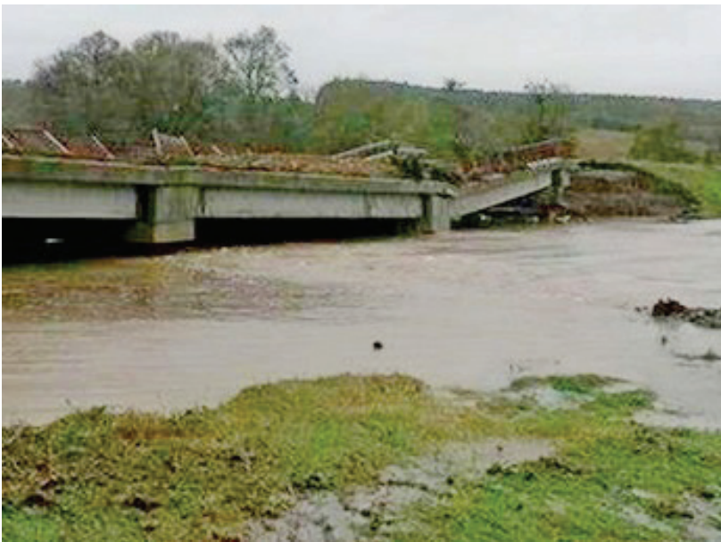
Figure 2. During the floods of September 2014, the bridge over the Ropotamo River near the village of Veselie collapsed during the torrent
